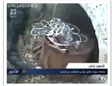
Syrian Rebels Test and Use Culvert IEDs.
