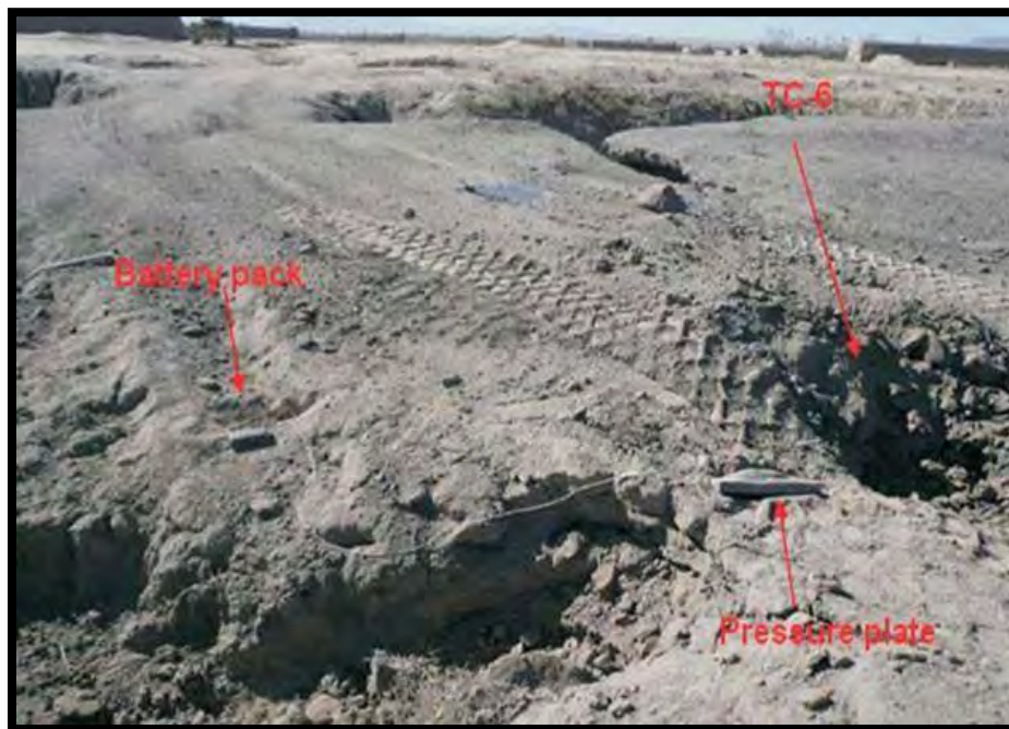
Figure 3-35 Danger Area- Washed Out Section of a Road
