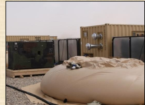
Pictured above is one 60K generator and 5,000 gallon water blivet needed to operate one double lane mobile wash rack.
