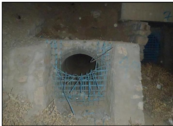
Partially open culvert denial systems should raise a red flag
