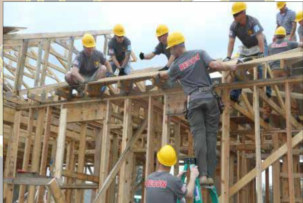
Soldiers assigned to 3rd Squadron, 1st Cavalry Regiment, 3rd Armored Brigade Combat Team, 3rd Infantry Division nail down the top of the roof during their ‘day of service’ with Habitat for Humanity, Columbus, Ga., Dec. 6. In addition to helping others, community service gives Soldiers a chance to enhance team building skills.
