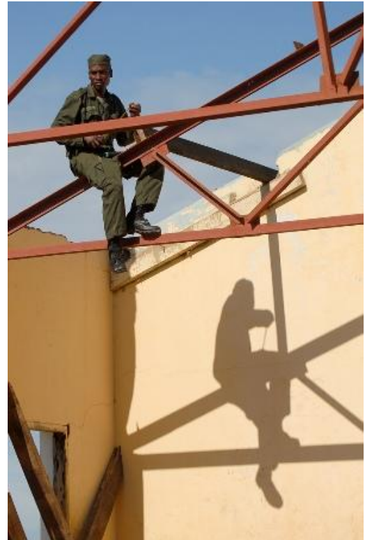
Figure 33 - The need for risk management is great; notice the lack of fall protection
