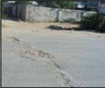
IED Buried in Pothole - Somalia
