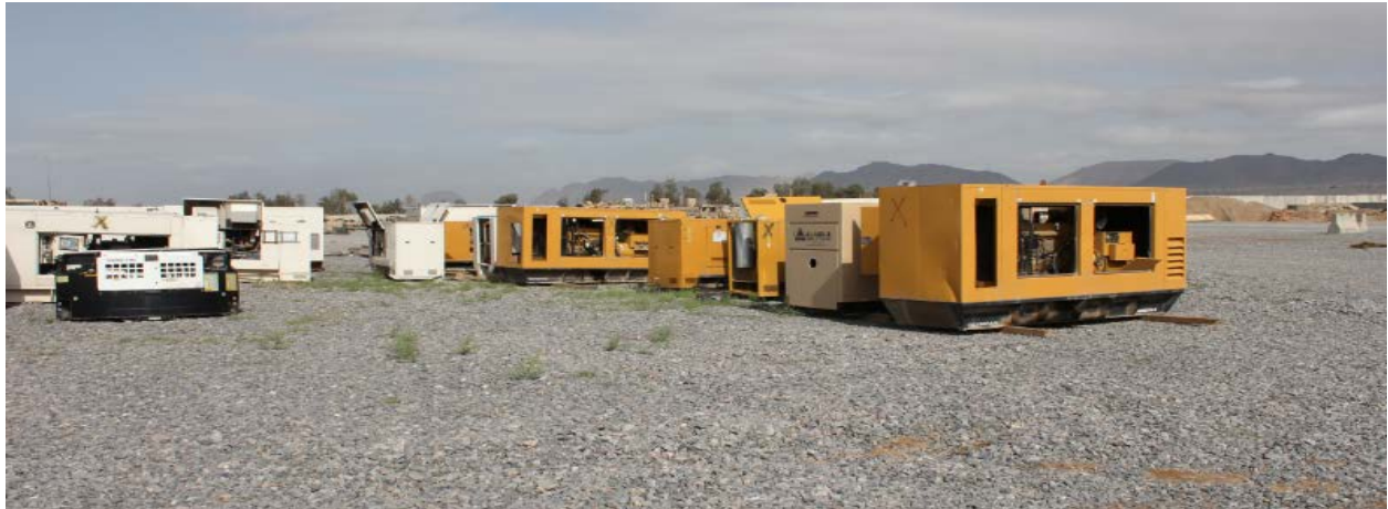
Figure 3: Generator storage yard with cannibalization
