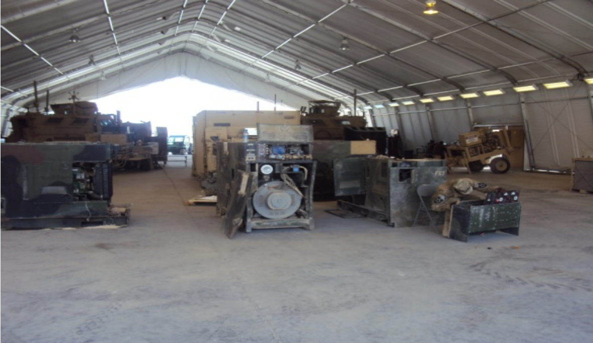
Figure 2: Generator Maintenance Bay
