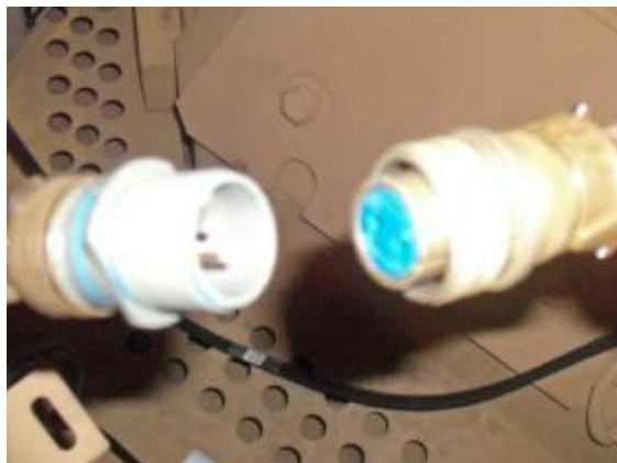
Figure 4-44. Dome Light Power Cable
