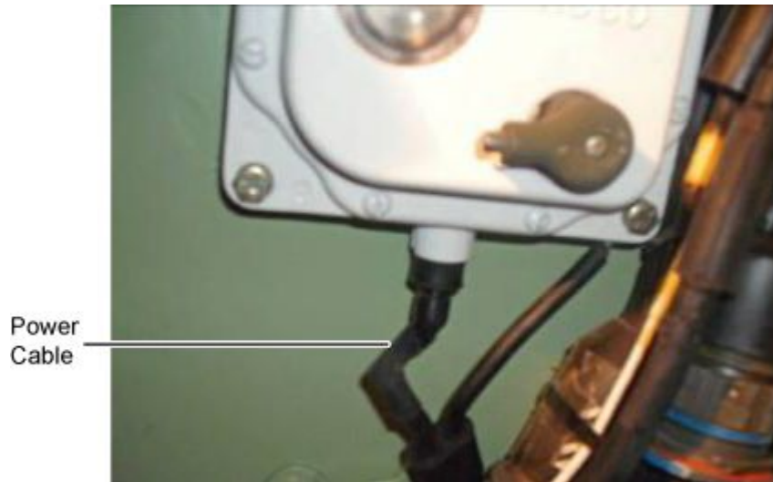
Figure 4-33. Dome Light Power Cable
