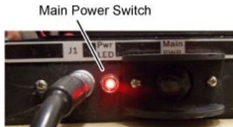
Figure 2-37. Main Power Switch
